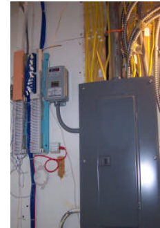
Dedicated Telecom and Electrical Service
